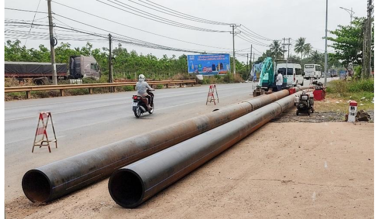
Underground drilling technology for pipeline development along National Highway 1A, Thong Nhat district, Dong Nai province
